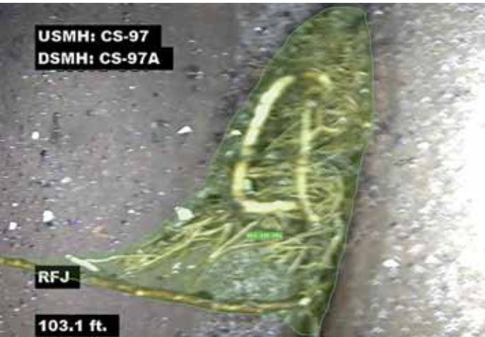
Figure 4. Screenshot from an updated video inspection file following an AI scan. The green overlay depicts Roots Fine Joint (RFJ) with an AI confidence interval of 92.2 percent. The text entries within the black box are video overlays from the certified operator where an RFJ at 103.1 ft (31.4 m) was indicated.
