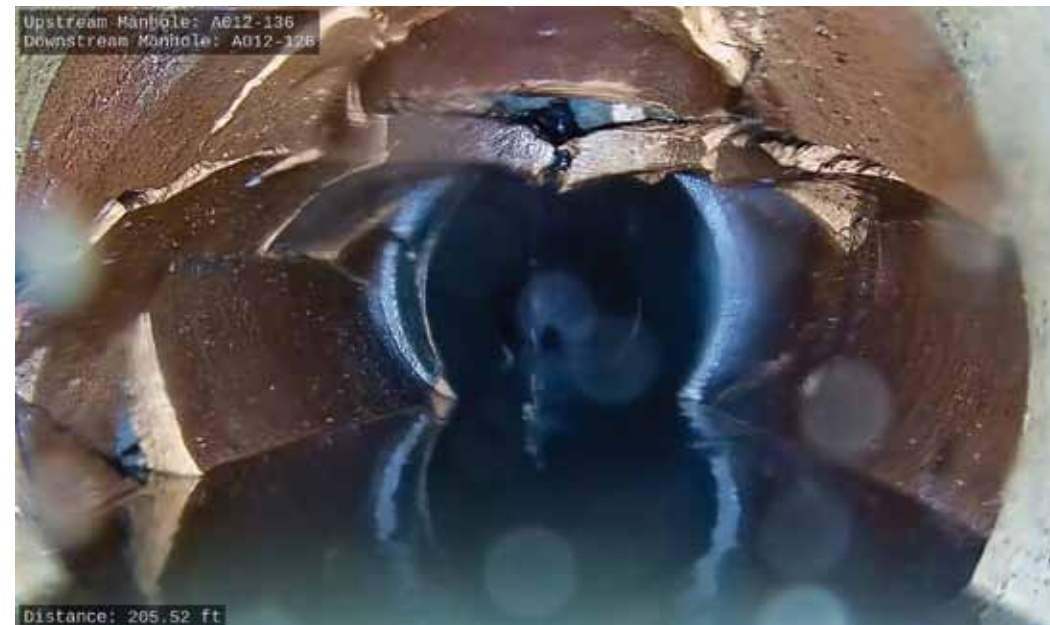
Figure 1. Sewer system evaluation surveys are comprehensive programs performed on gravity sewers to target structural defects and infiltration and inflow entering the system
