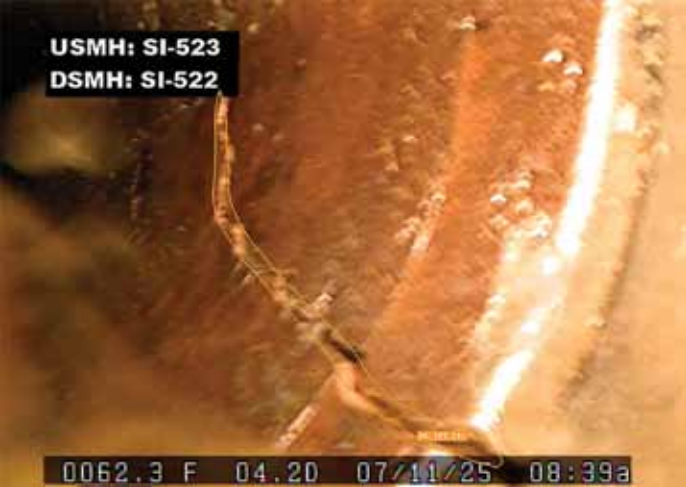
Figure 6. Screenshot from an updated video inspection file following an AI scan. The orange overlay depicts Fracture Longitudinal (FL) with an AI confidence interval of 97.1 percent.
