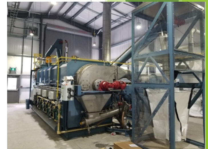
CHAR Technologies High Temperature Pyrolysis
