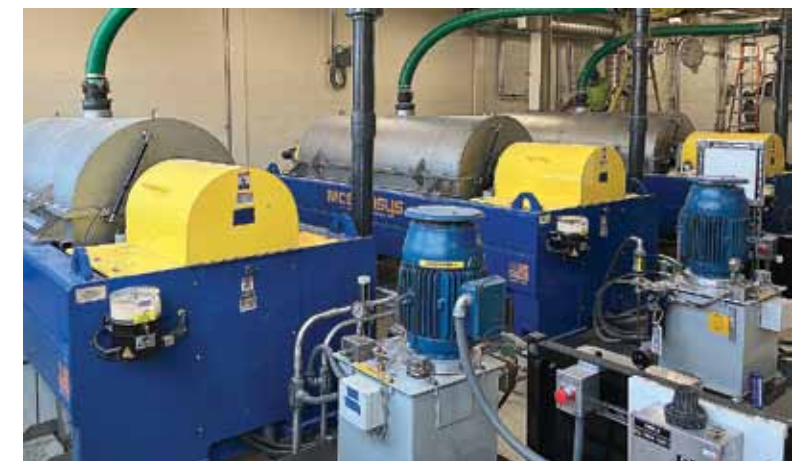
Photo 4. Thickening centrifuges in WAS thickening room
