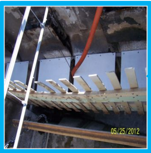
Sludge Protector Baffles
