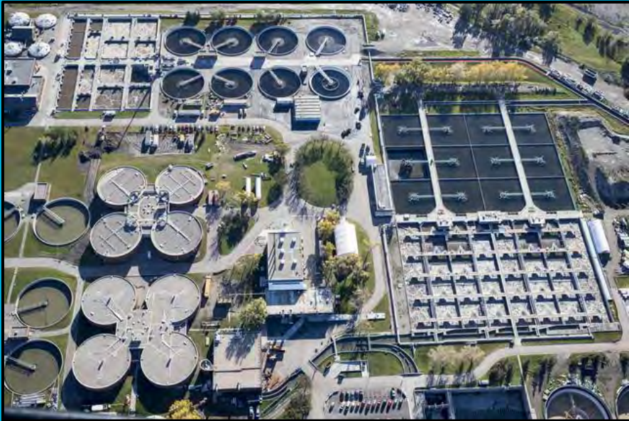
Aerial photo of the Grand Rapids wastewater treatment plant along the Grand River. (City of Grand Rapids)
