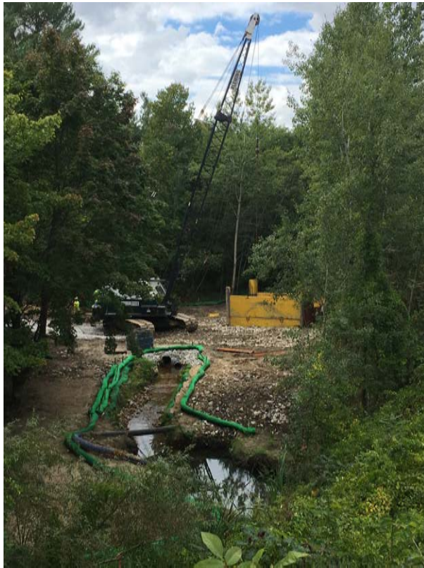
Prior to Restoration
