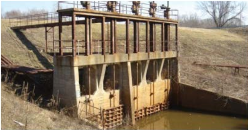
Floodplain Storage and Flood Walls (Hartford, CT)
