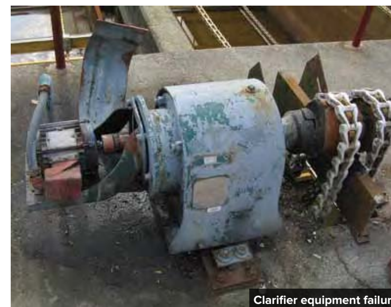
Aeration equipment failure
