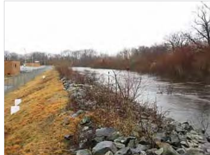
This levee, which protects the Warwick WWTF, was breached on March 30, 2010, flooding the treatment plant area
