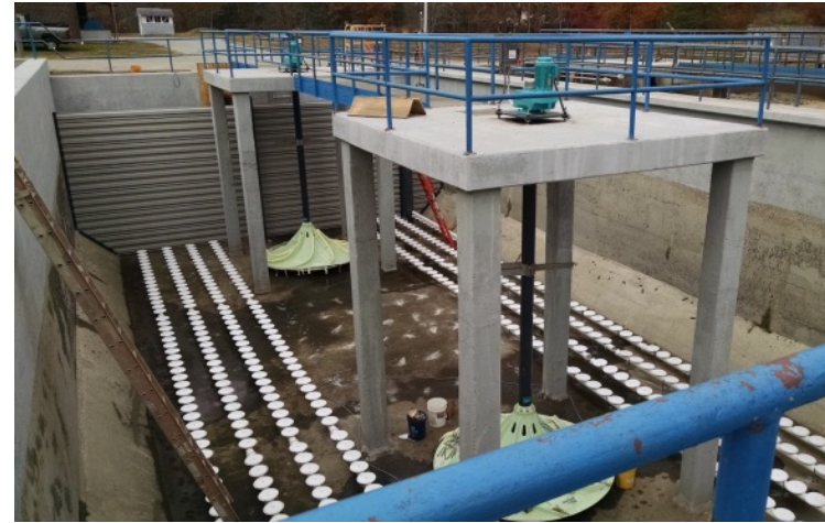
New Diffused Aeration
