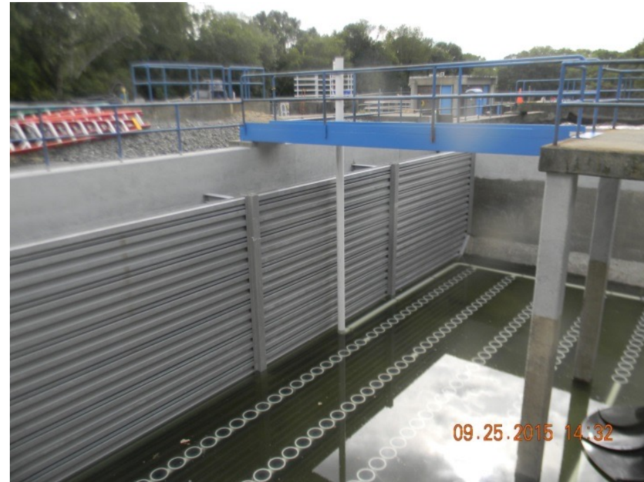
New Biological System On Line
