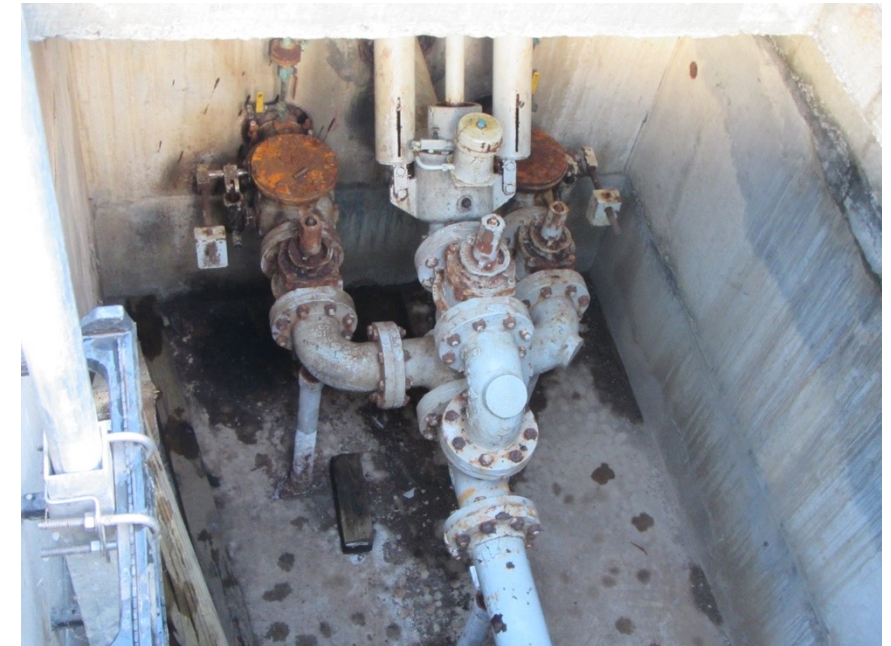
Pump Station Valve Vault
