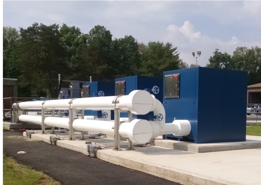
New Blowers and Aeration Piping
