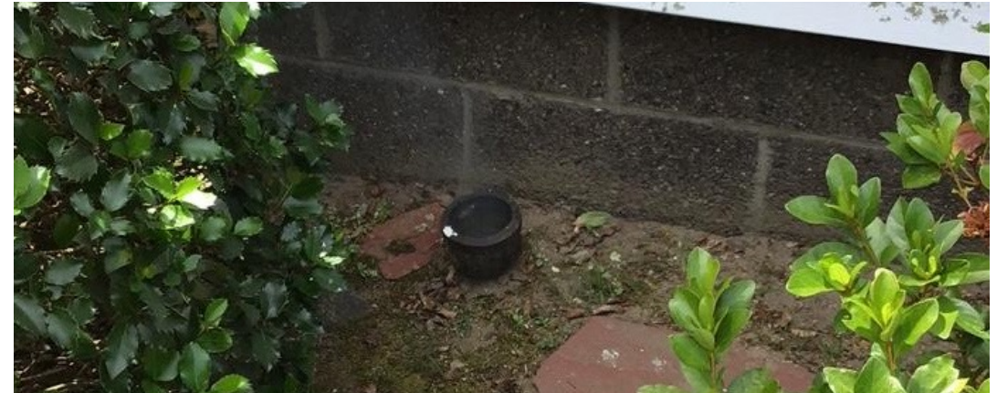
9 Defective or Missing Cleanouts (Mostly in Separated Areas)
