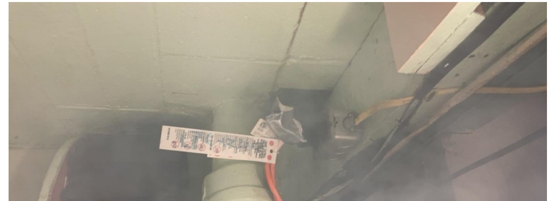
20 Potential Illicit Connections from Homes/Structures/Buildings (Mostly in Separated Areas)
