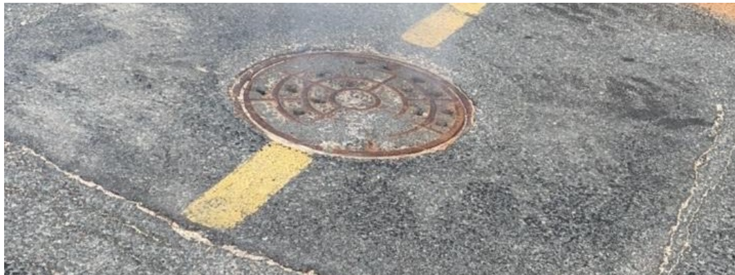
31 Vented Manhole Covers (50/50 in Separated vs. Combined Areas)
