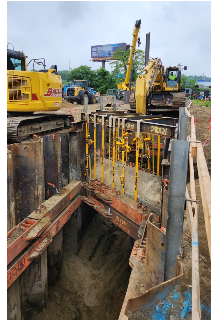
Work Required Supporting the 48- Inch Mill River Relief Sewer in Place SRA Property
