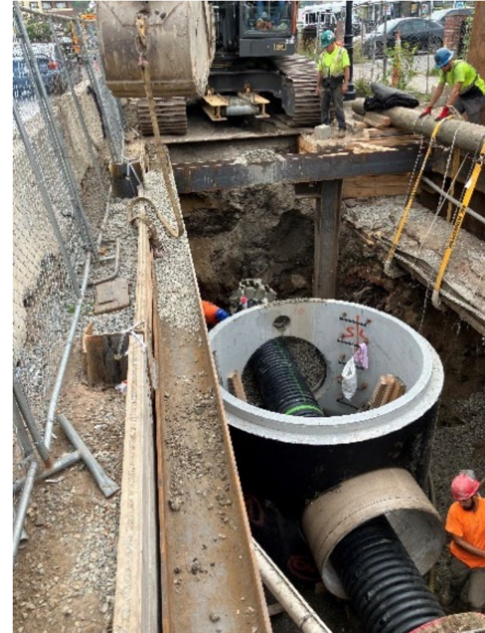
Temporary Flow Conveyance with ADS Pipe for Wet Weather Contingency Main Street
