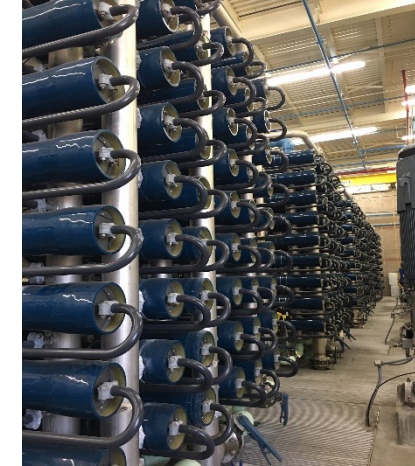
Nanofiltration/Reverse Osmosis (NF/RO)
