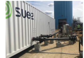
Figure 1: SUEZ specialty ion Exchange container used to remove PFAS in the drinking water supply
