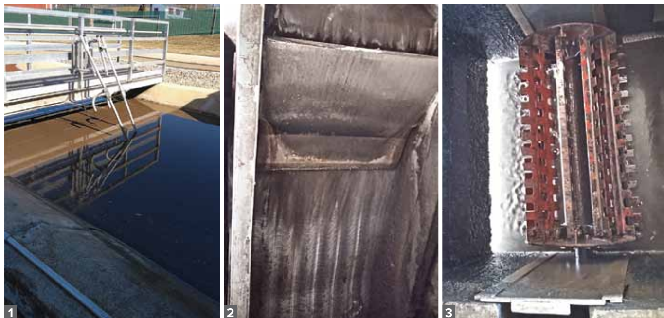
1. Dissolved oxygen and oxidation reduction potential probes in oxidation ditch 2. Influent screen 3. Original drum aerator
