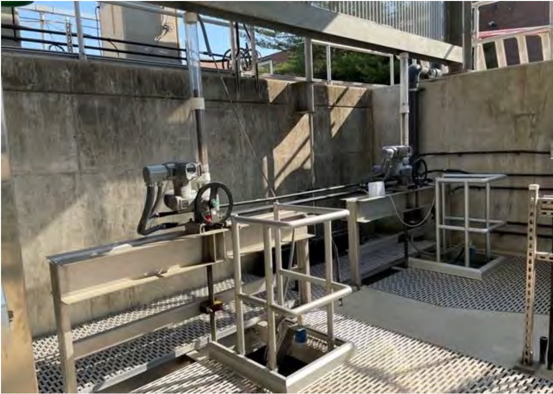
Directly measure flow over UV channel effluent weir gates
