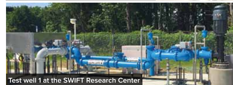
SWIFT pilot at the York River Treatment Plant
