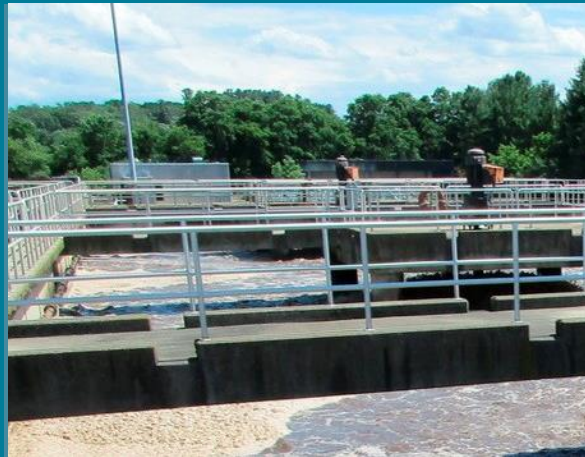
Haverhill, MA Water & Wastewater
