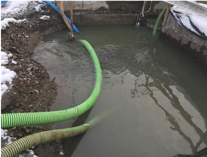
Initial leak at air release structure
