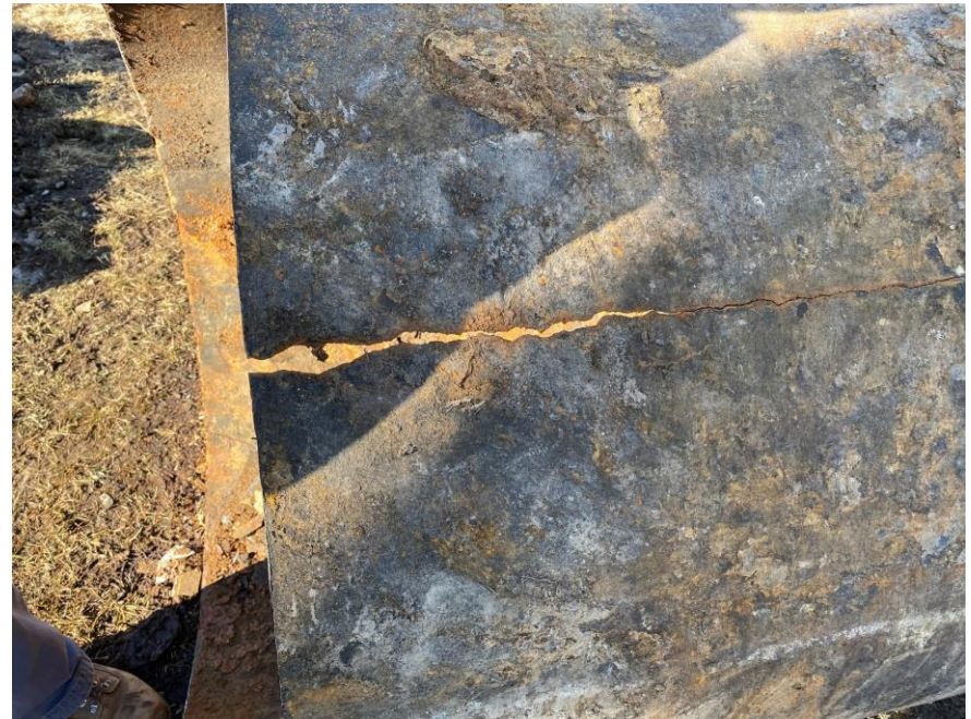
Longitudinal crack in 42-inch pipe
