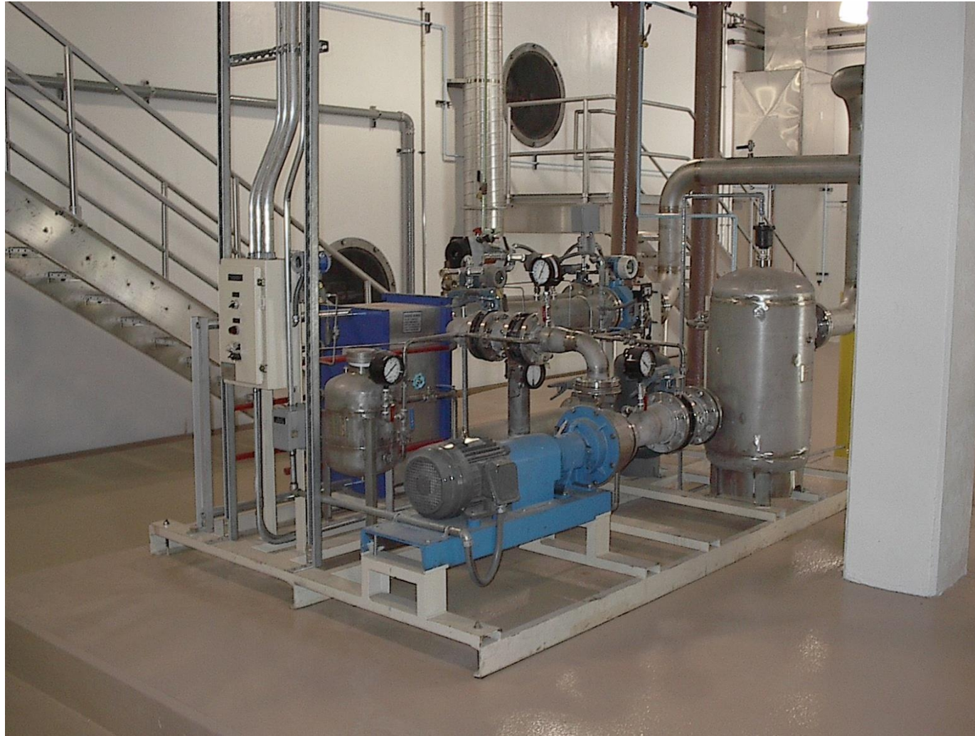
Closed Loop Cooling Water System Sky Lake WTP - Orlando, FL
