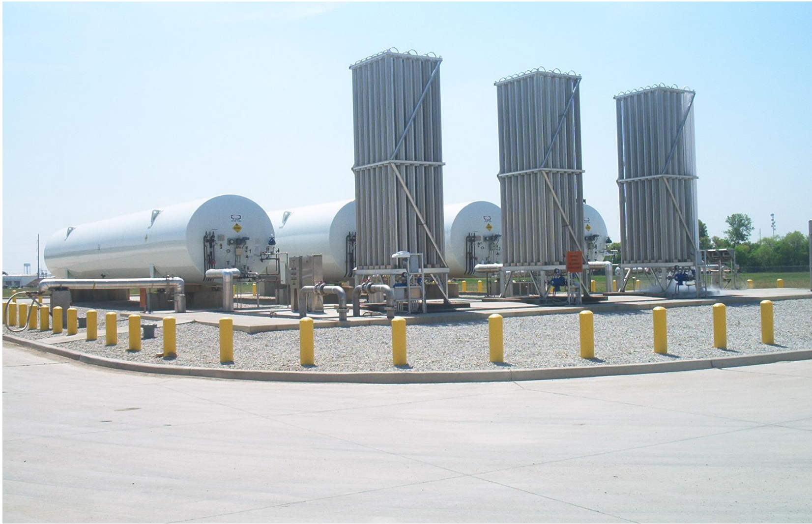
LOX System – Fort Worth, TX – Rolling Hills WTP
