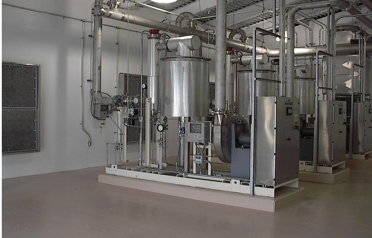
Ozone Destruct Units 3 x 300 CFM Sky Lake WTP
