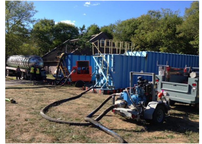
Emergency Response to FM Break
