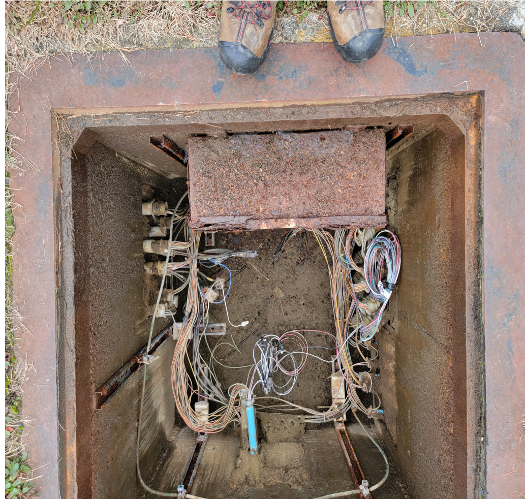
Yard Electrical Distribution
