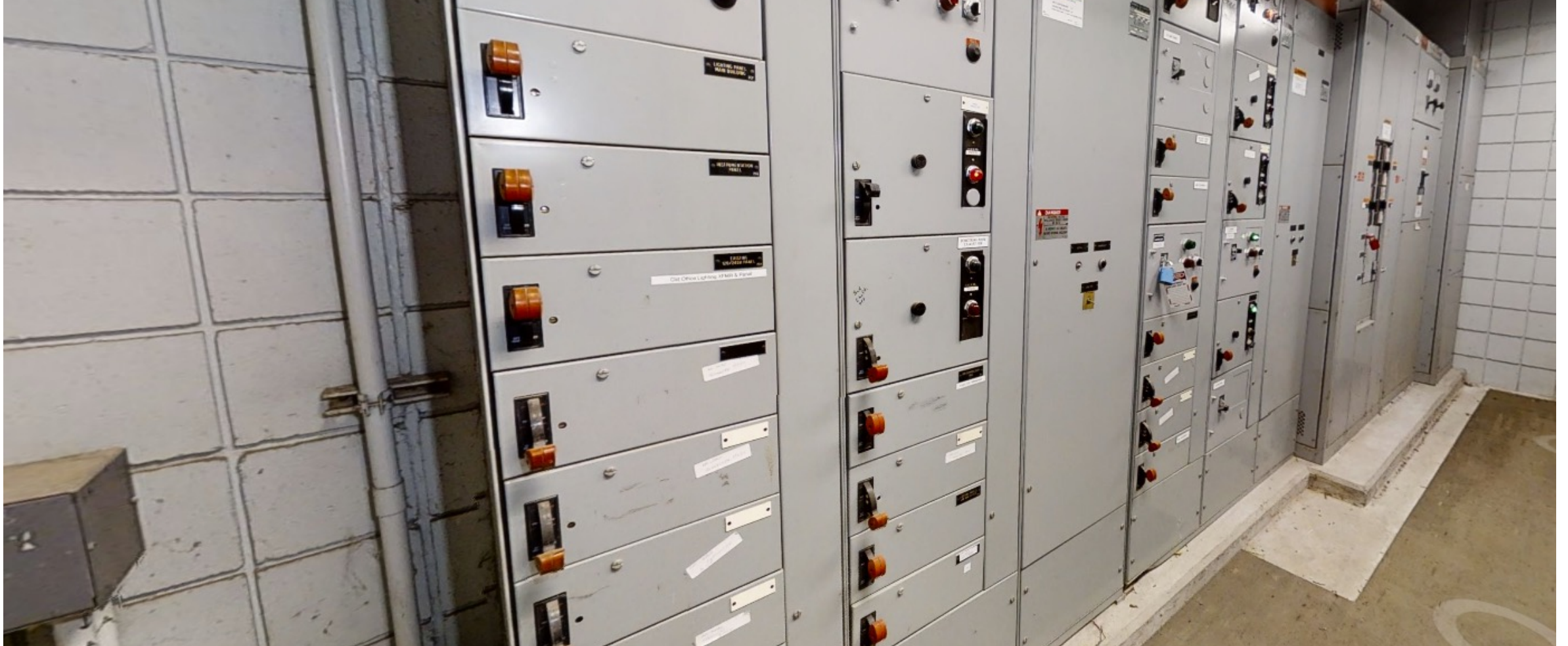
Motor Control Center (1988)
