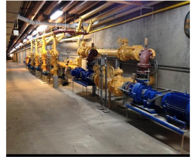
Transfer & Mix Pumping Station
