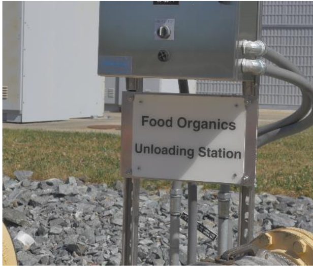
Truck Offload Stations
