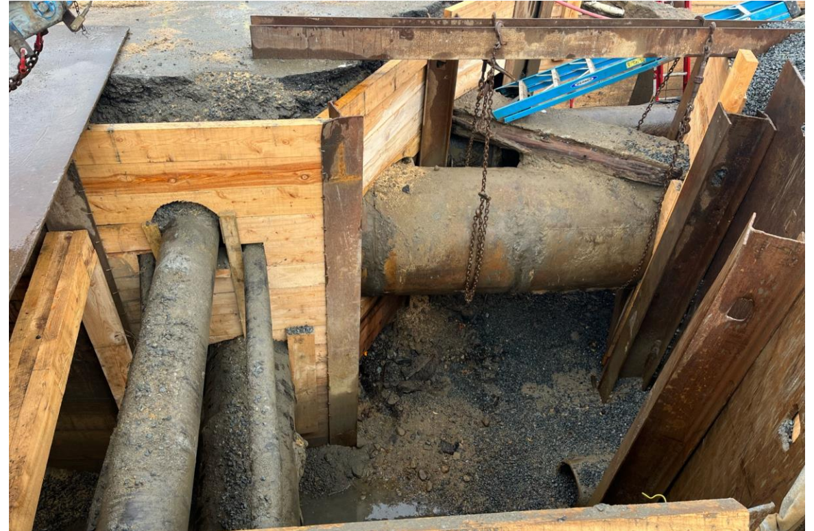
Custom trenching required due to large quantity of utilities in the Lynnway
