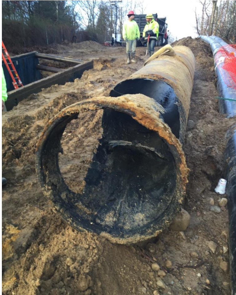
Break due to Hydrogen Sulfide
