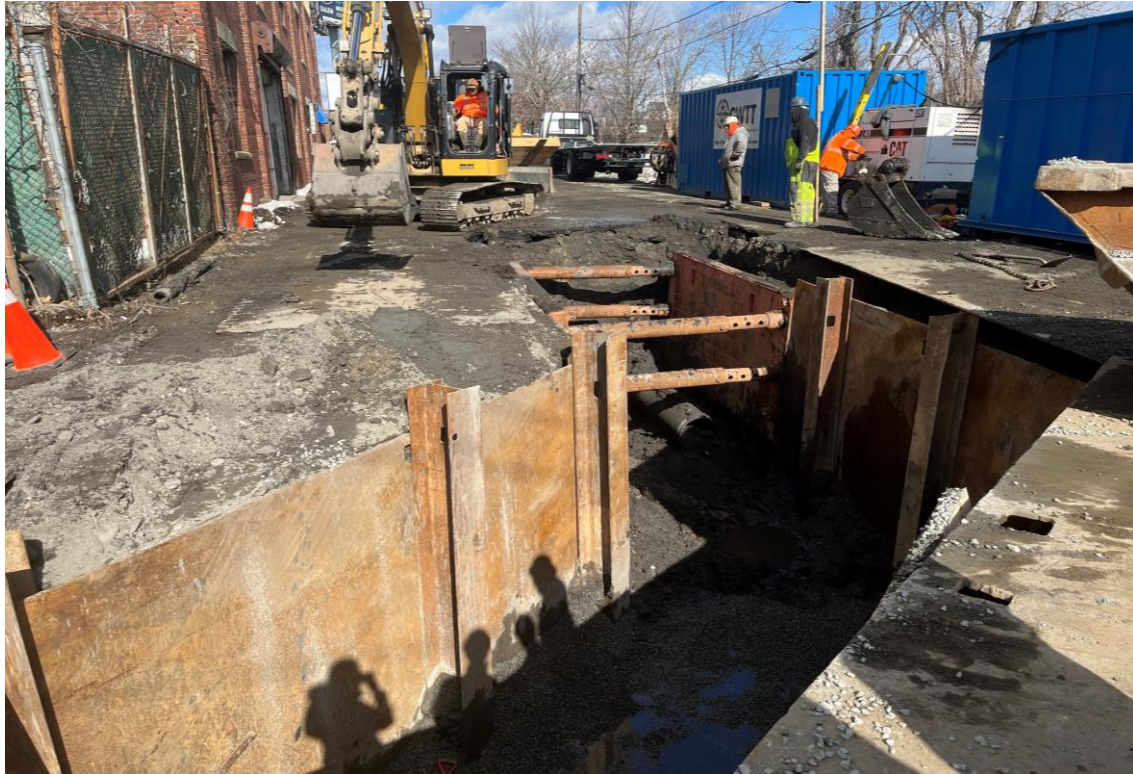
Contaminated groundwater and soils uncovered during excavation
