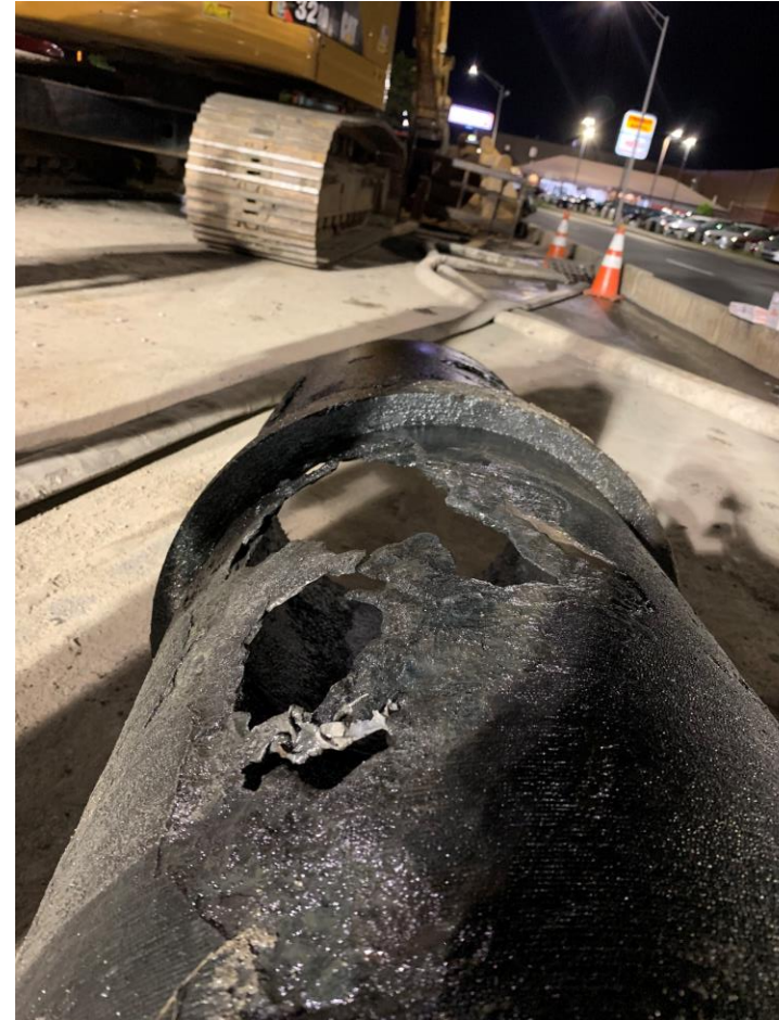
Break caused by Electrolic (Stray Current)
