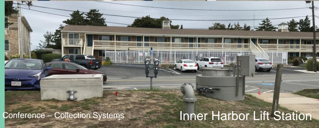
Falmouth Beach Lift Station
