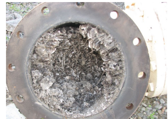
Digested sludge piping elbow
