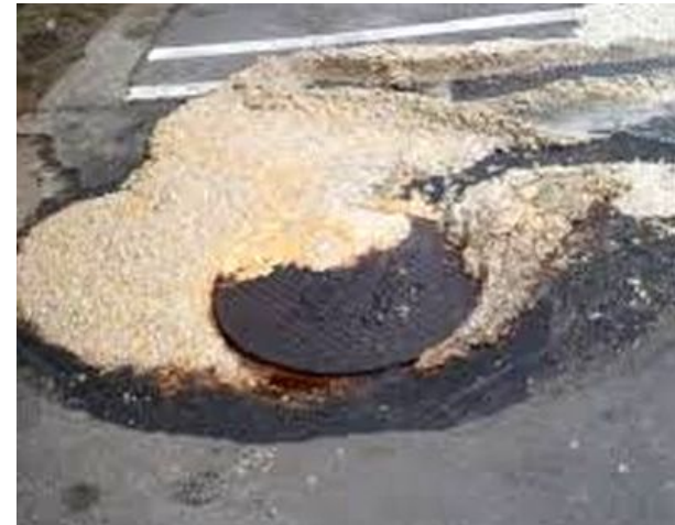
Sanitary Sewer Overflow
