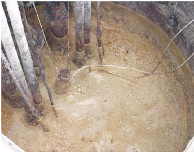
Choked Pump Station
