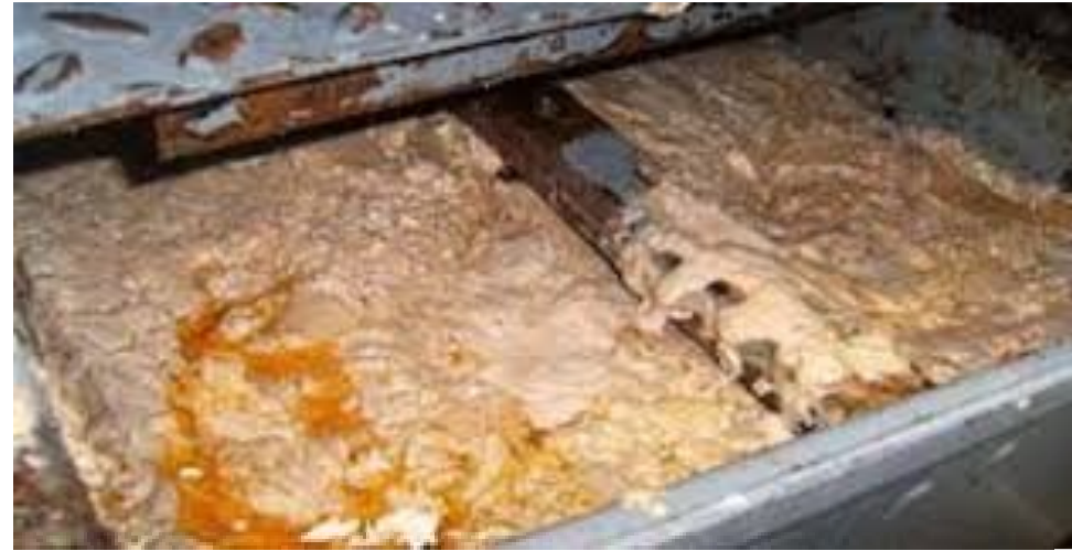
Neglected Grease Trap
