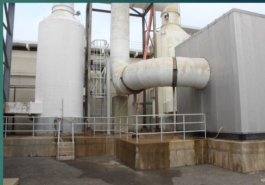
Odor Control Facility A Scrubbers and Fan Building
