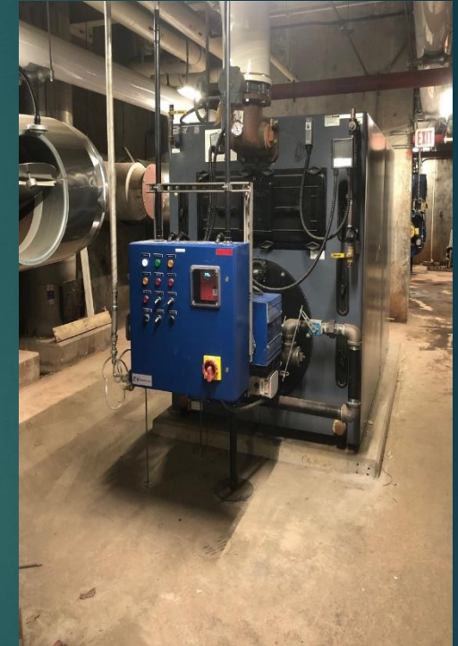
New 5MM Btu/hr Hot Water Boilers
