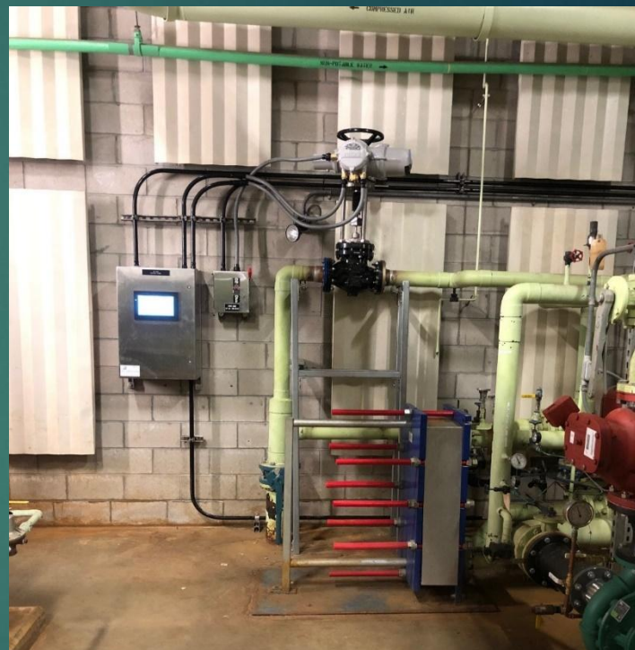
Process Cooling Water Control Valve
