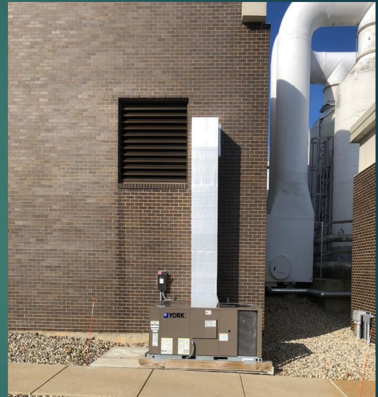
Example of Outdoor HV Unit
