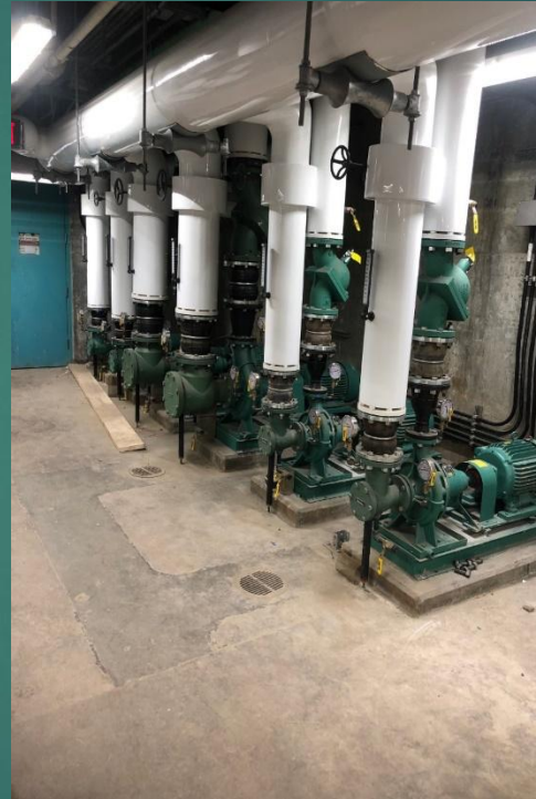
New Hot Water Recirculating Pumps
