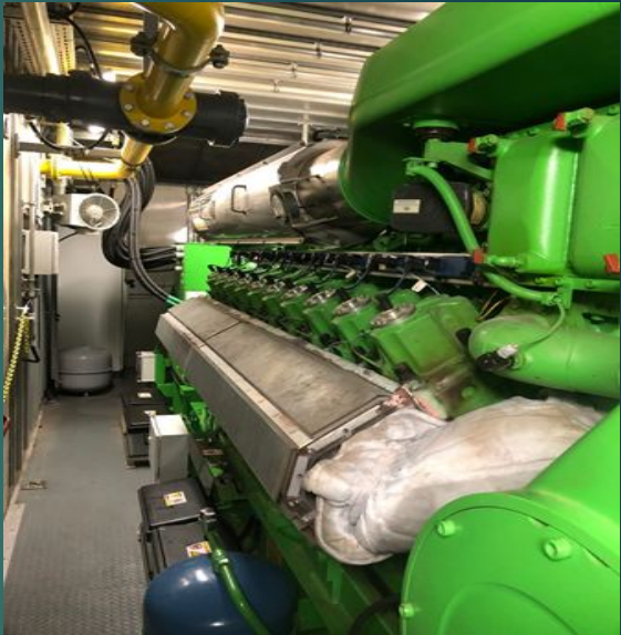
1.4 MW CH&P Engine Generator
