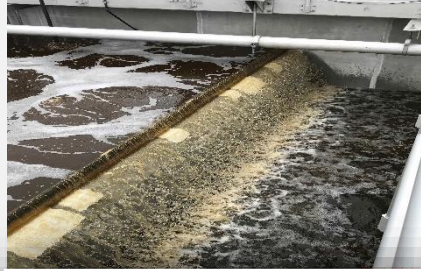
Post Aeration Zone
