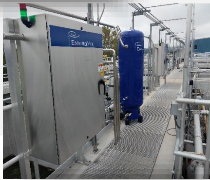
Compressed Gas Mixing (CGM) System
