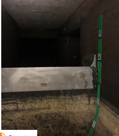
View of weir and measurement visual from camera
