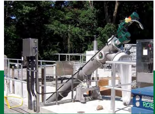
New Hartford WWTP, Hartford, CT
