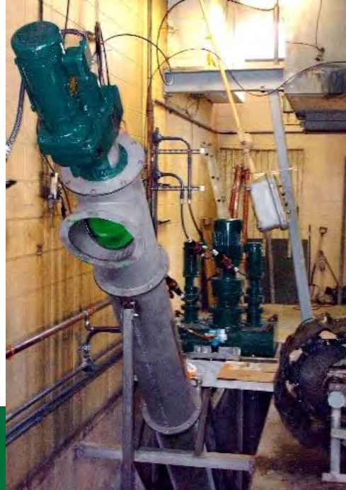
Manchester WWTP, CT
