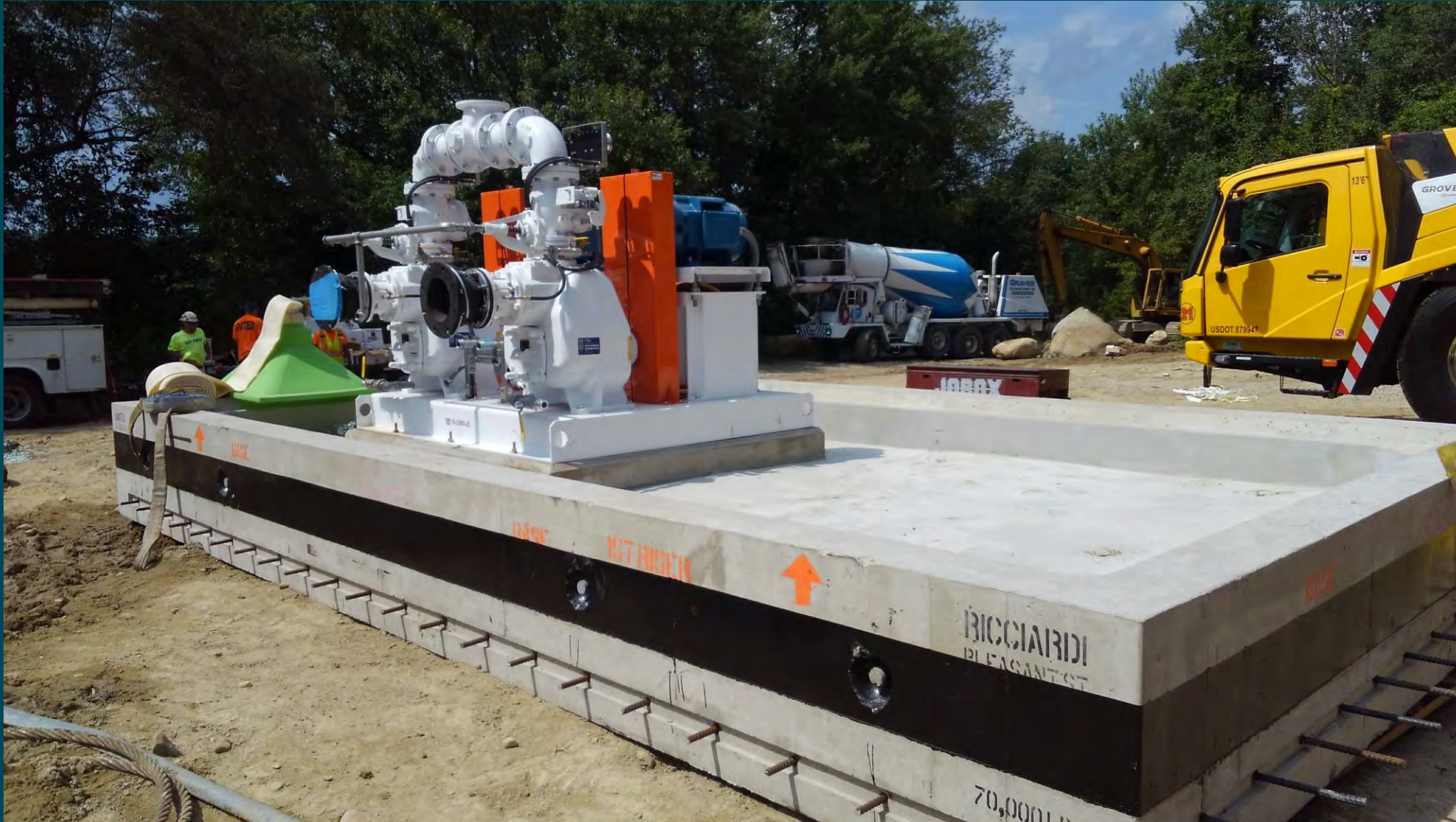
Gorman-Rupp Pump Skid on Slab
