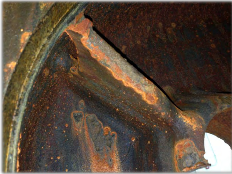
Damaged Pump Casing
