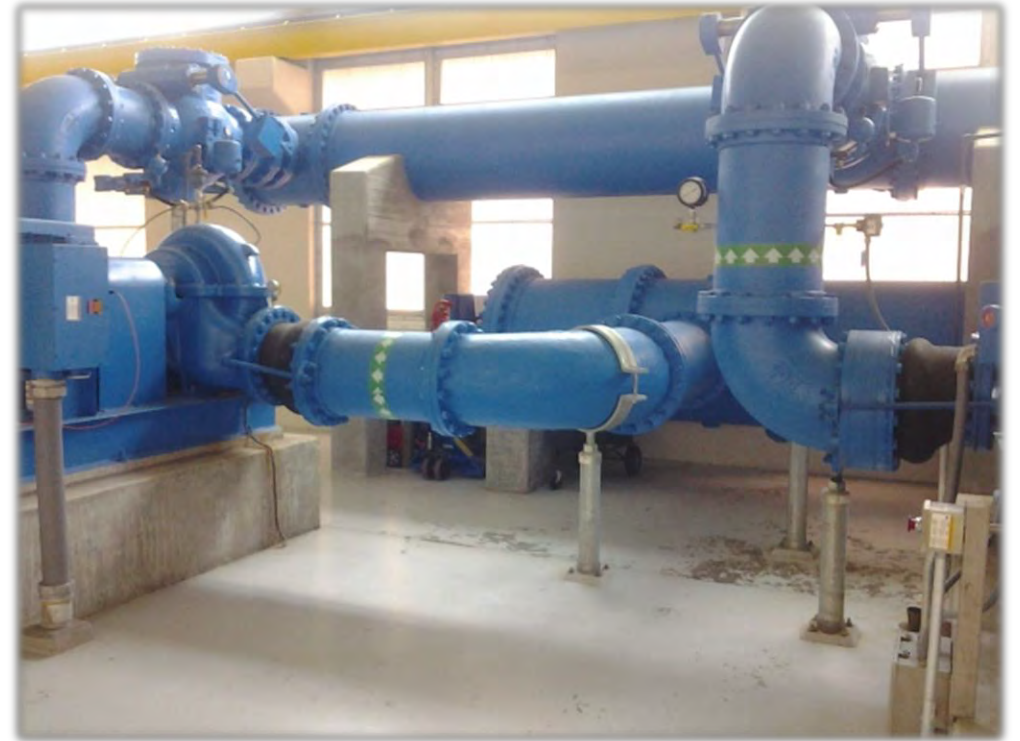
Existing Suction Piping
