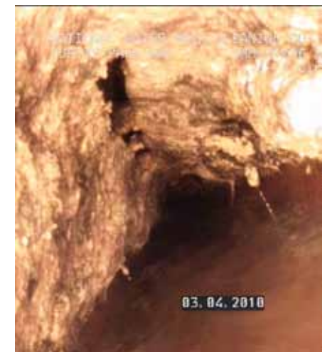
Grease buildup recorded during CCTV inspections in Webster Square
