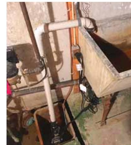
Sump pump connected to sewer system
