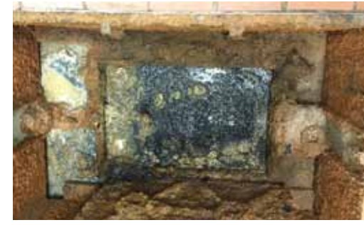
Grease trap not properly maintained between the two inspection periods
