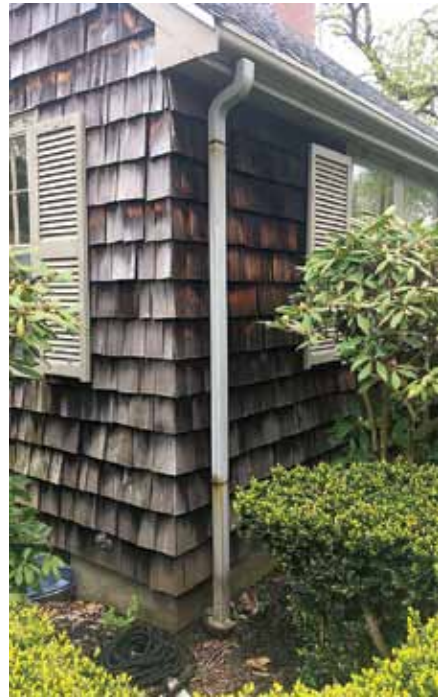
Roof drain connected underground
