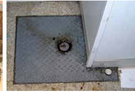
Walk-in freezer built over the floor unit grease trap, preventing maintenance
