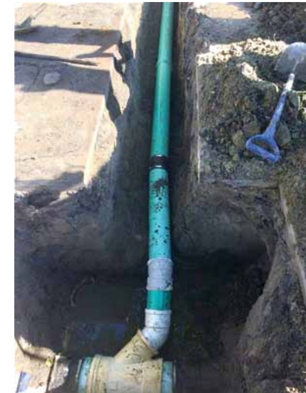
Redirection via a direct drain pipe connection
