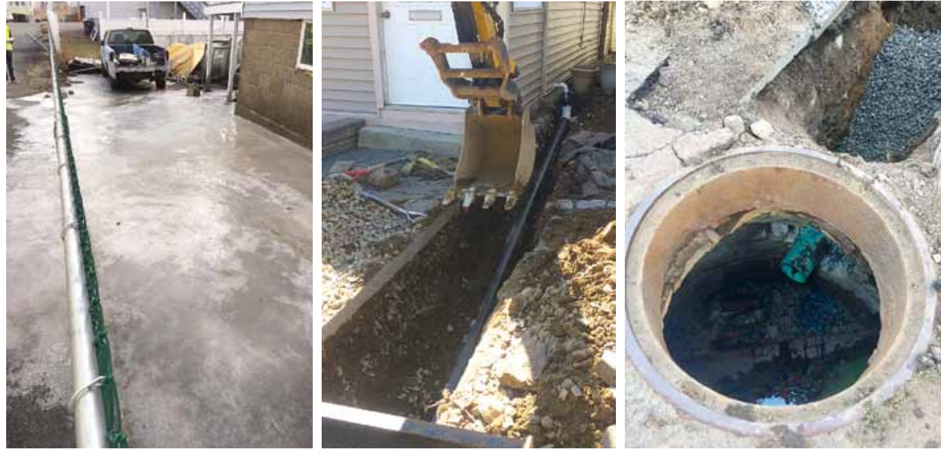
Sump pump ice hazard
