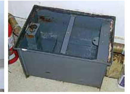
Clean grease trap with proper sizing and venting
