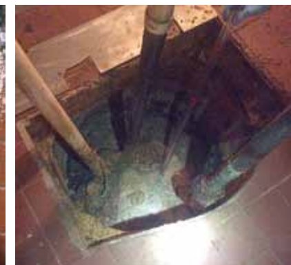
An open pit filled with grease found during one of the inspections
