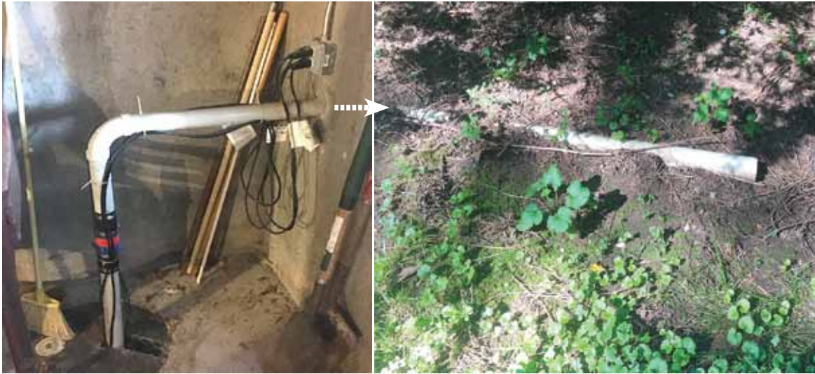
Properly installed sump pump system
