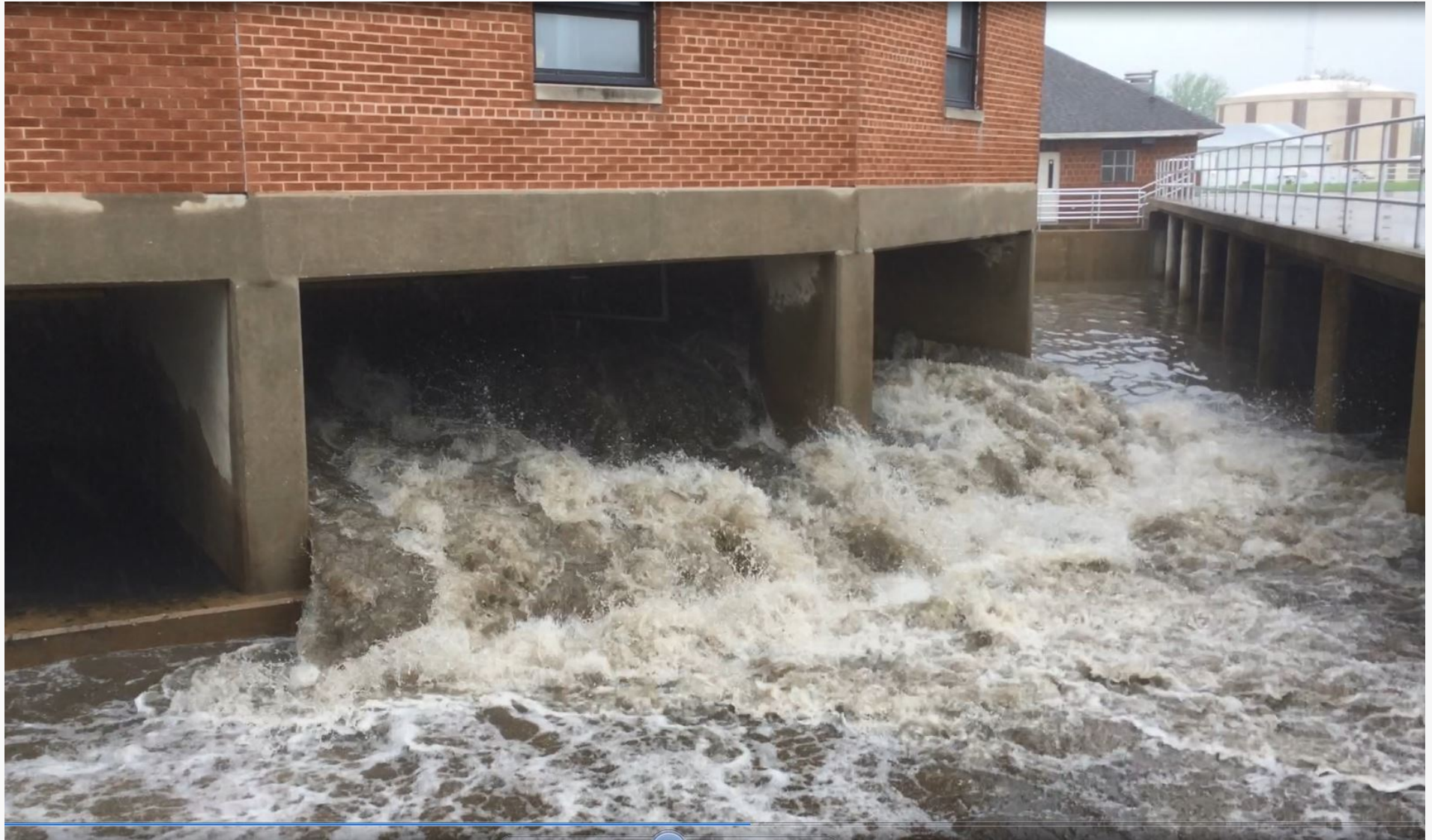
PUMP No. 5 IN OPERATION
