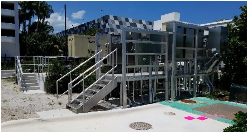
Elevated roads and pump station
