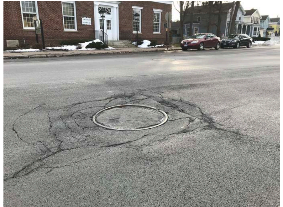
Traditional Frame & Cover Road damage after 2 years
