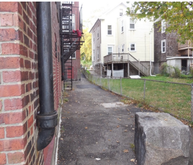
Building Roof Drainage - Downspouts
