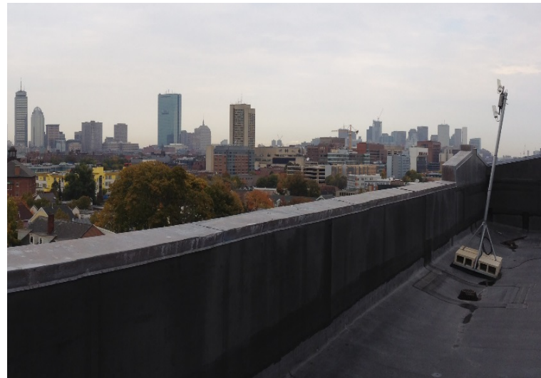
Building Roof Drainage - Internal
