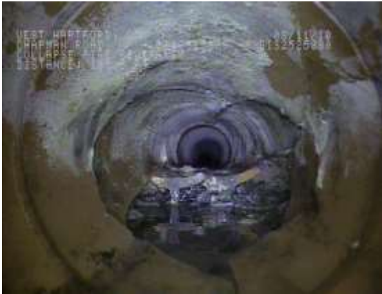
Sewer Main Defect
