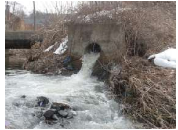
Sanitary Sewer Overflows
