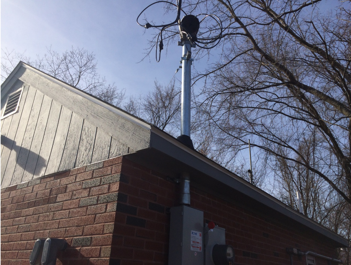
New Electrical Service w/ Weatherhead (East Natick I PS)
