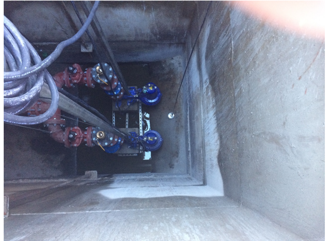
New Submersible Pumps @ East Natick II PS
