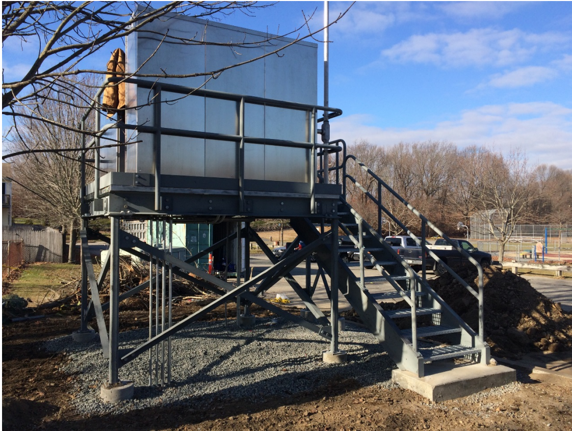
Elevated Steel Platform @ East Natick II PS
