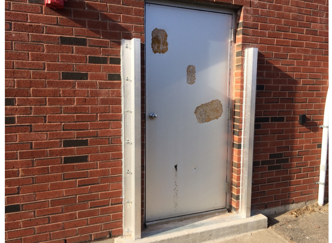
New Door Flood Barrier Channels (East Natick I PS)
