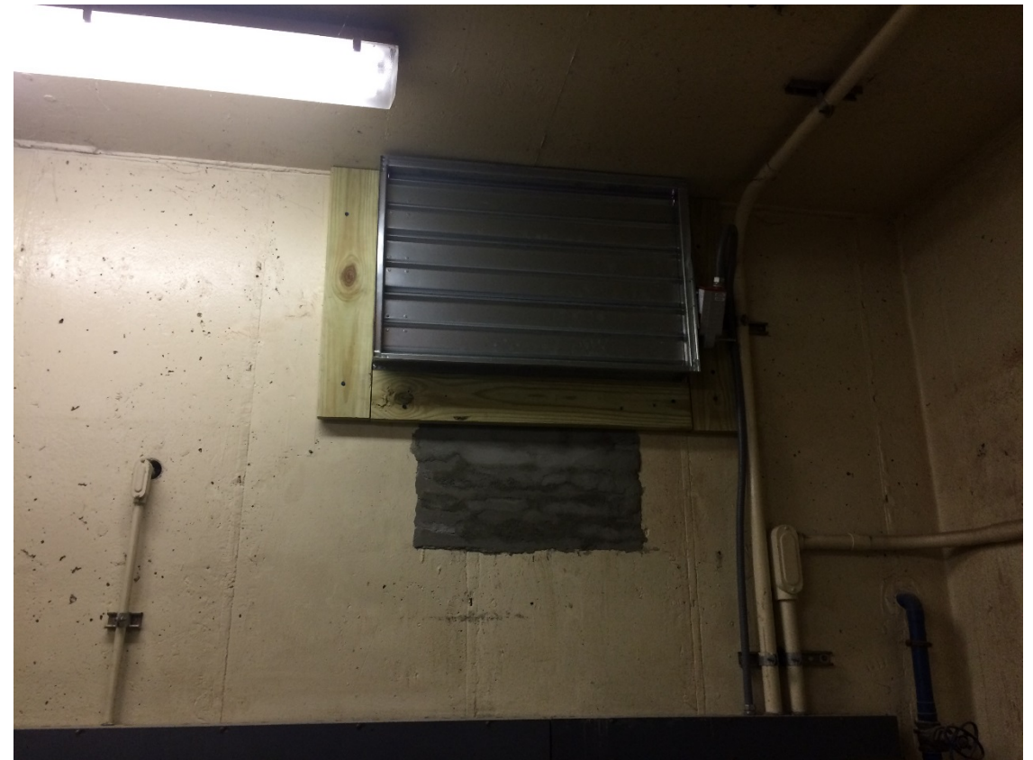
Interior View of Relocated Intake Louver (East Natick I PS)
