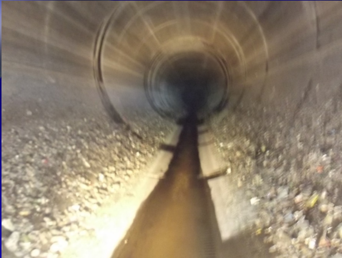
Debris on Sides of Tunnel
