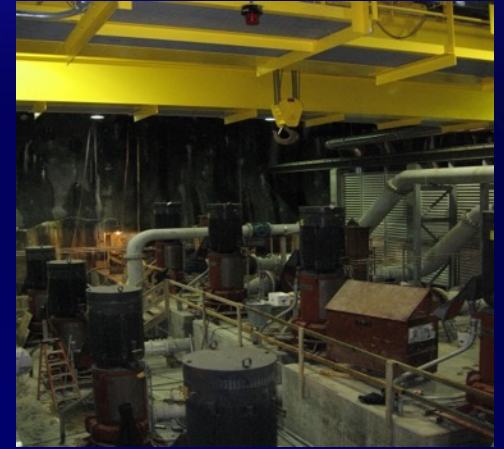
Tunnel Pump Station 2,500 pieces of equipment
