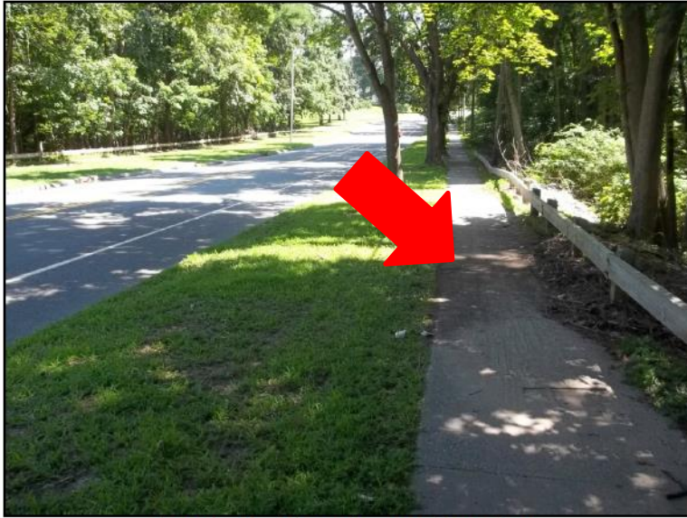
Route 5 sidewalk overtopping
