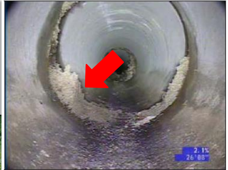
Sand leaking through pipe joints on Willow Brook Rd.
