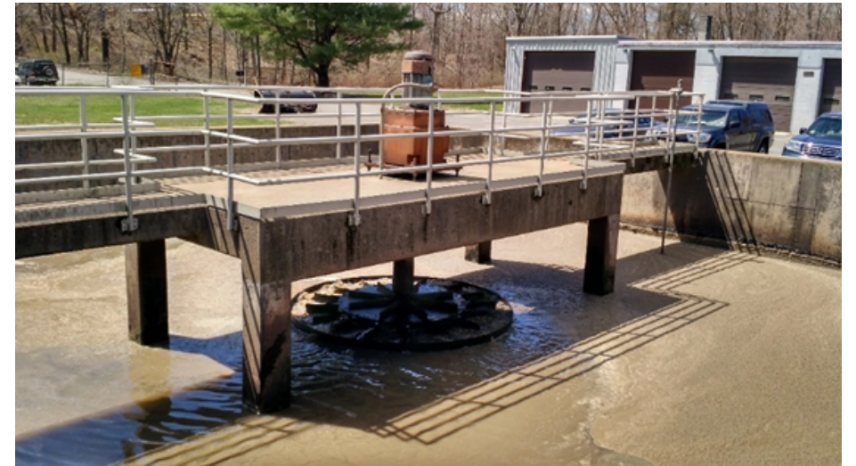
Existing Mechanical Surface Aerator
