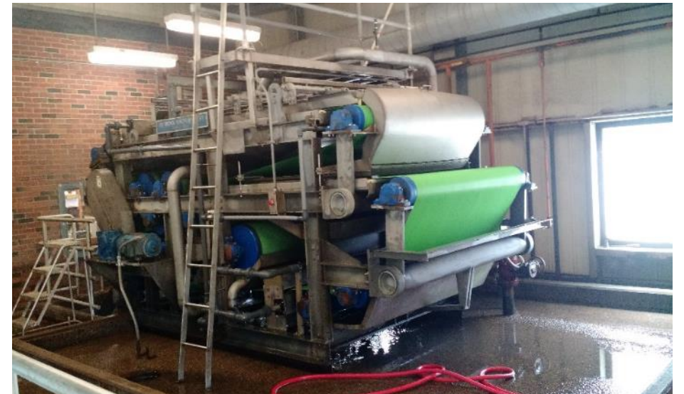
Existing Belt Filter Press
