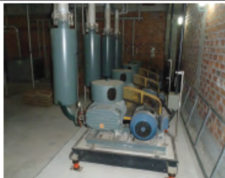
Waste water Treatment Facilities in Aeon Mall
