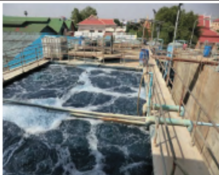
Wastewater Treatment Facilities in Dye House
