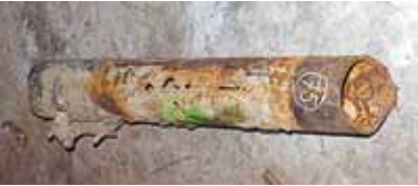
Figure 3. Corroded cast iron pipe
