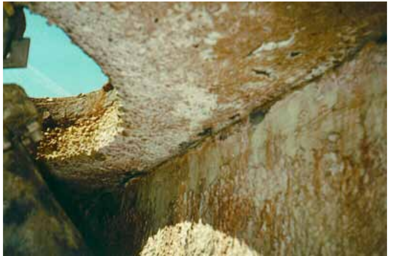
Figure 5. Biogenic sulfide corrosion/vapor phase, five years of exposure
