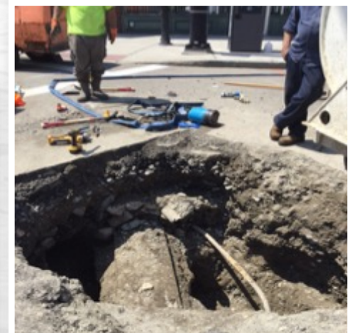
Avoid Street Collapse
