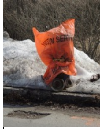
Hydrant—Out of Service
