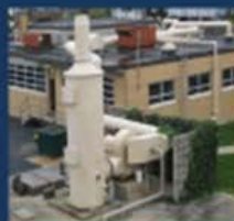
11. Replace worn odor control system fans and control panel
