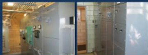
8. Replace worn electrical service/transformers, equipment, and lighting
