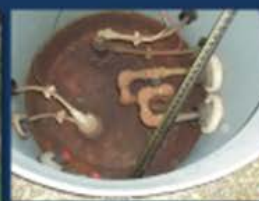
12. Replace worn underground fuel storage tanks and piping
