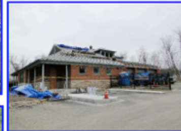
"A" Street Waste Water Management Facility
