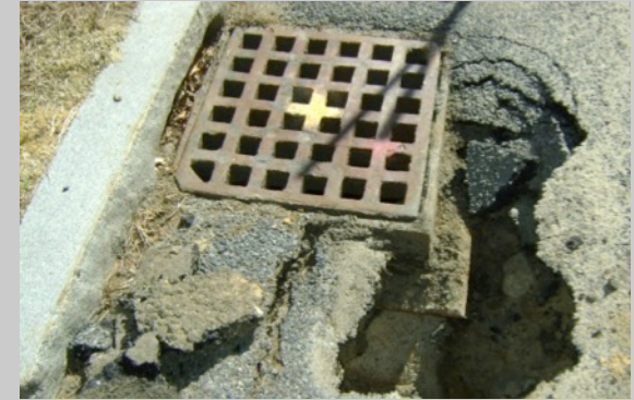
Sink hole forming near catch basin
