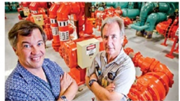
PHOTO: Site Services engineer Art Kierle (left) and mechanic Doug Macpherson helped replicate water and cost savings from Kent, Wash., to El Segundo, Calif. KATHLEEN M. SPICER/BOEING
